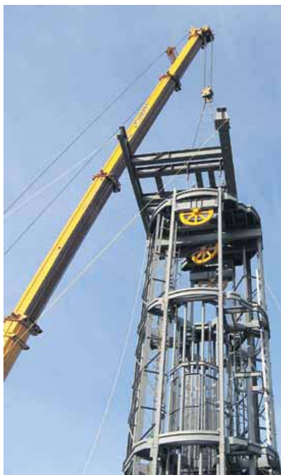
A crane lowers a galloway, a working platform that can have several working decks, into a mine shaft to continue the sinking process.
